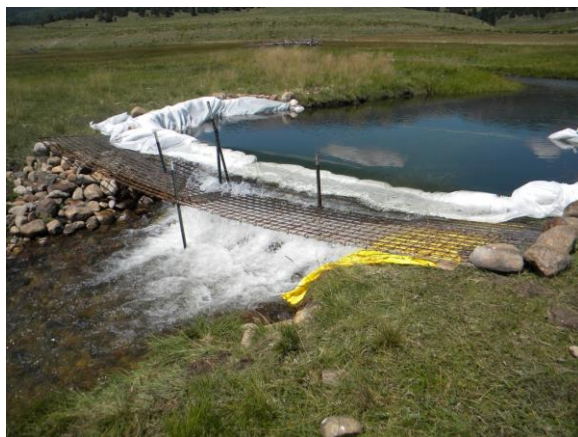
Fig. 12.4. A seasonal fish migration barrier on Costilla Creek. This barrier was installed in July to prevent fish moving out of Costilla Reservoir and into treated stream reaches prior to reservoir treatment in October. The barrier was removed from the stream following reservoir treatment.
