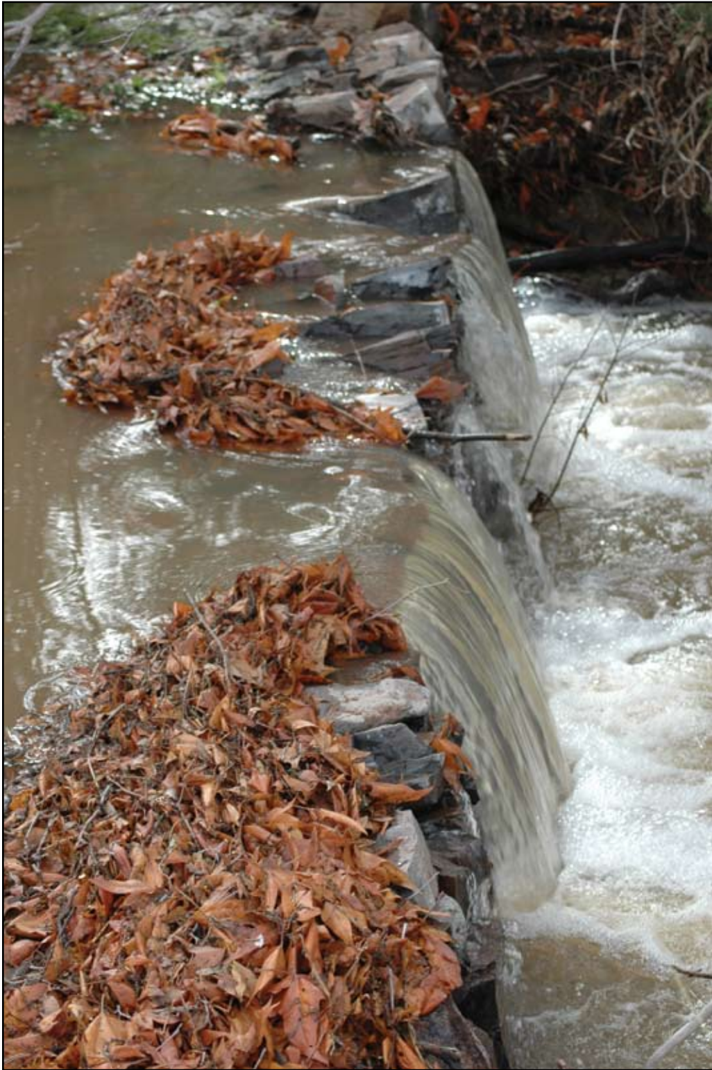
Loose rock structure with flowing water.
